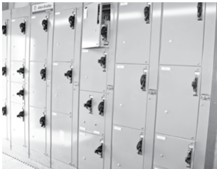
One of four electrical stations
